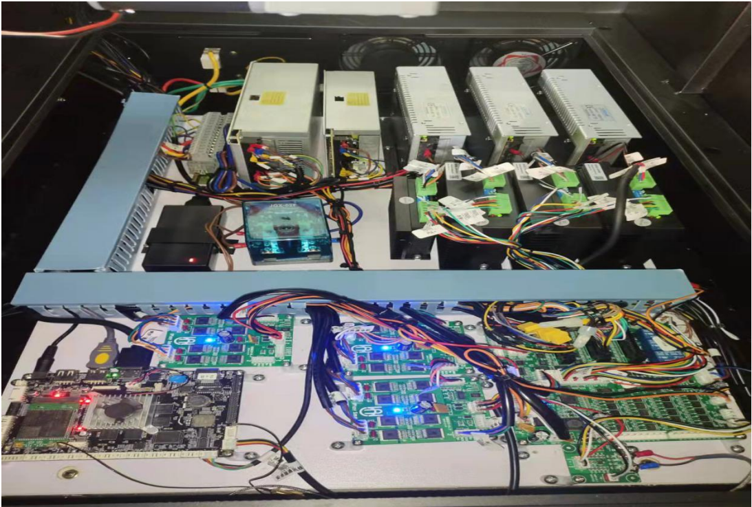
The main control room is located in a steel box directly below the oven
